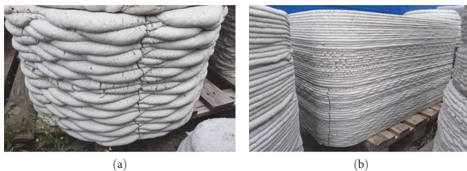
FIGURE 9: Cracking results of concrete products 3D printed. (a) Continuous slit in a product with a round cross-section with a bottom. (b) Continuous slit (in the lower part) in a hollow product with a bottom.
